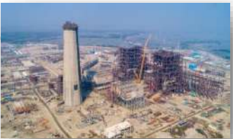
2X660 MW at Rampal, Maitree, Bangladesh-BIFPCL
